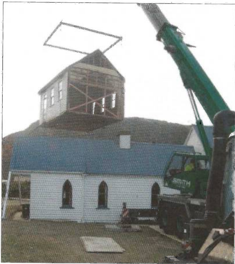
The Millers Flat Church ascends towards the heavens on the first stage of its miraculous journey to, probably, its final resting place, near Provisions Cafe, at Adam's cottage.
